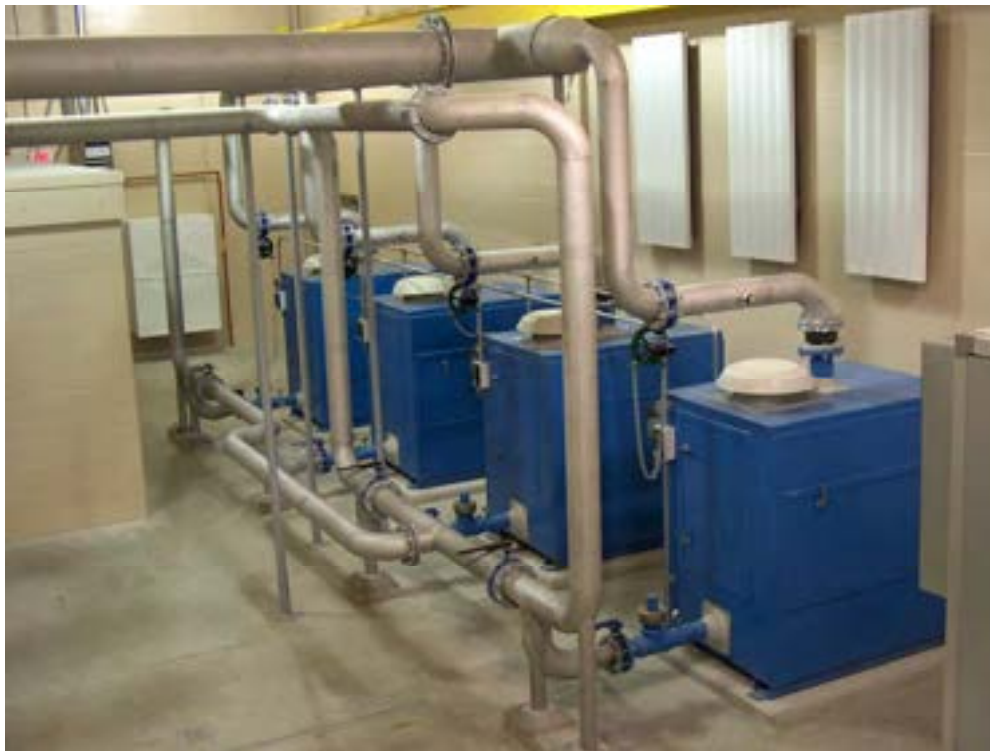
Four ThermAer ATAD blowers, 3 duty blowers with 1 stand-by
